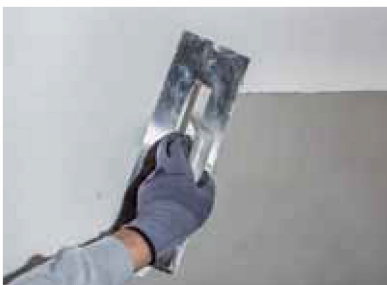
Figure 1 İstanbul Mavi Mineral Textured Decorative Plaster is applied on the surface with trowel.
