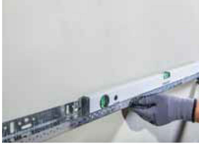
Figure 1 In the first step of the application; gaps, indentations, and protrusions between the wall and the İstanbul Mavi Socle Profile are corrected using wedges of varying thicknesses, and the surface is measured with a surface level.
