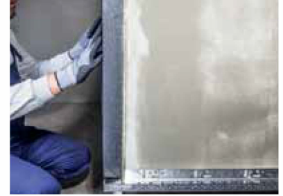
Figure 3 The dimensions of the socle profiles, which should be mounted with a gap of 2-3 mm between them, are selected based on the thickness of the thermal insulation board to be used.
