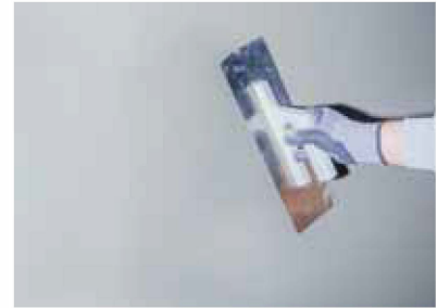
Figure 3 Application of the second layer of the plaster mortar is completed after waiting for slight dehydration of the first layer depending on weather conditions.
